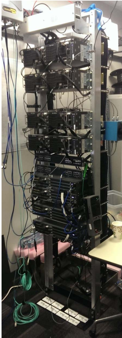
Figure 1 - Staged 9500 MPR Rack in Test Lab
