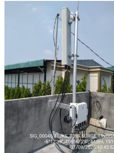
Wall-mounted South Jakarta
