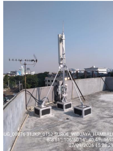
Ballast-mounted guyed pole Central Jakarta
